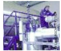
image FIRST GEOTHERMAL POWER STATION IN GERMANY PRODUCING ELECTRICITY. WORKER IN THE FILTRATION ROOM.
