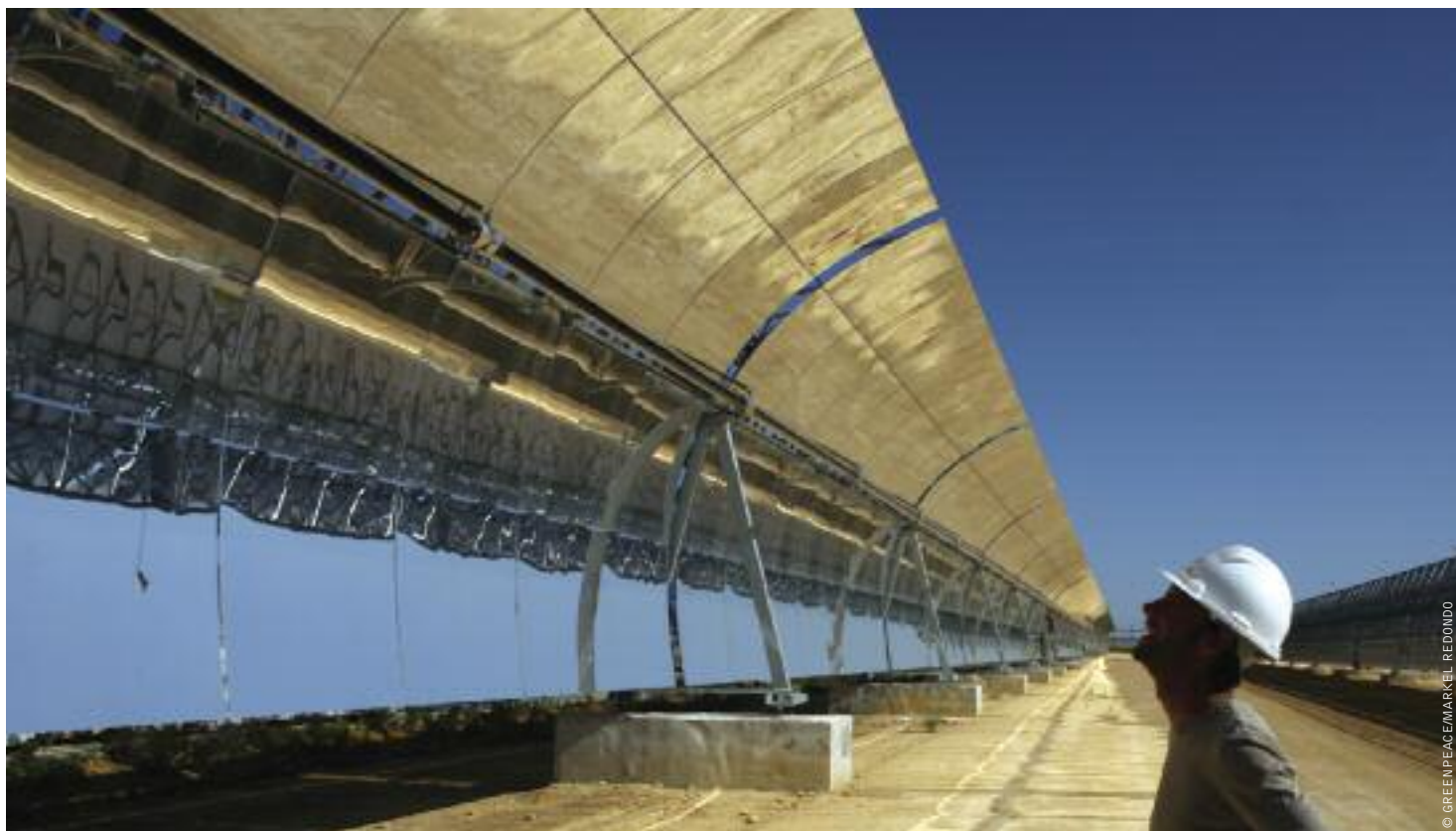
image WORKERS EXAMINE PARABOLIC TROUGH COLLECTORS IN THE PS10 CONCENTRATING SOLAR TOWER PLANT IN SEVILLA, SPAIN. EACH PARABOLIC TROUGH HAS A LENGTH OF 150 METERS AND CONCENTRATES SOLAR RADIATION INTO A HEAT-ABSORBING PIPE INSIDE WHICH A HEAT-BEARING FLUID FLOWS. THE HEATED FLUID IS THEN USED TO HEAT STEAM IN A STANDARD TURBINE GENERATOR.
