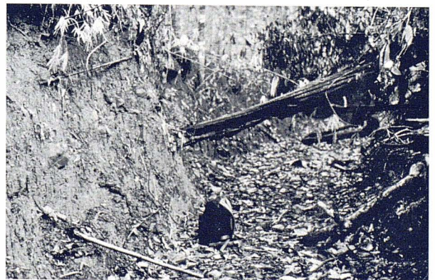
Figure 2. Erosion gully 3-4 m deep cut through colluvial deposits south-west of Doi Khu.
